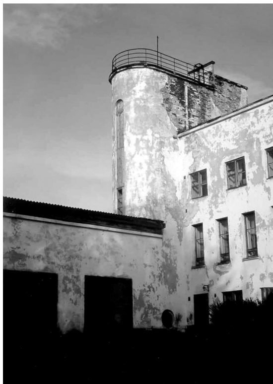
Fig. 3. The architecturally most remarkable building from the Finnish era in Border Karelia is the communal house and fire station in the former Suvilahti (present-day Suojärvi) now accommodating a kindergarten and a youth club. The building complex, built in a mature functionalistic style, with white stuccoed exterior walls, incorporating a semicircular tower, etc., was designed by architect Erkki Koiso-Kanttila, who was involved with the post-Winter War reconstruction, and completed during the Continuation War (1943). (Photo Netta Böök, 2001).
