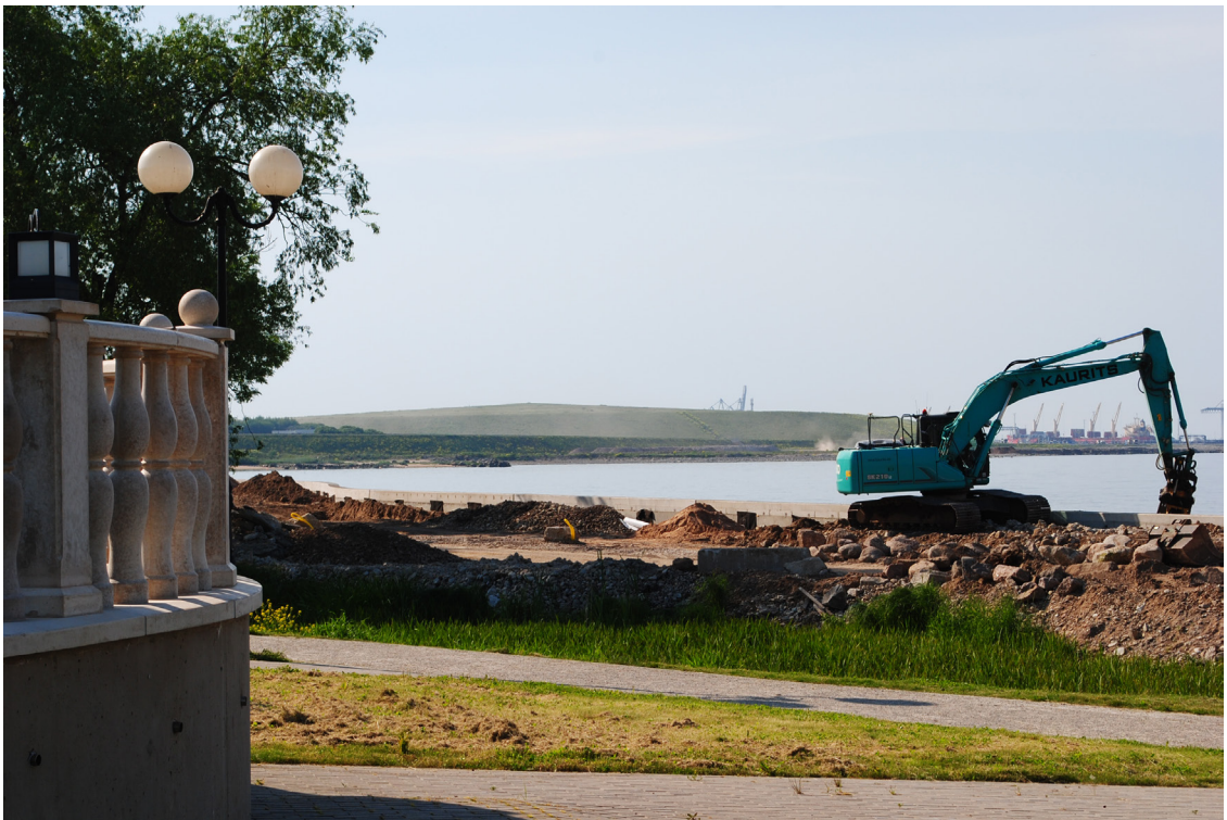
Fig. 1. The waterfront promenade under construction, with the radioactive waste hill in the background, Sillamäe, Ida-Viru, Estonia (Photo: Pikner 2020).
